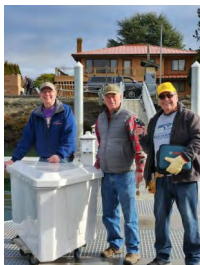
(Left to Right) Volunteers Tom Madden, Rick Parnell, and Ron Fortier installing dock boxes.
